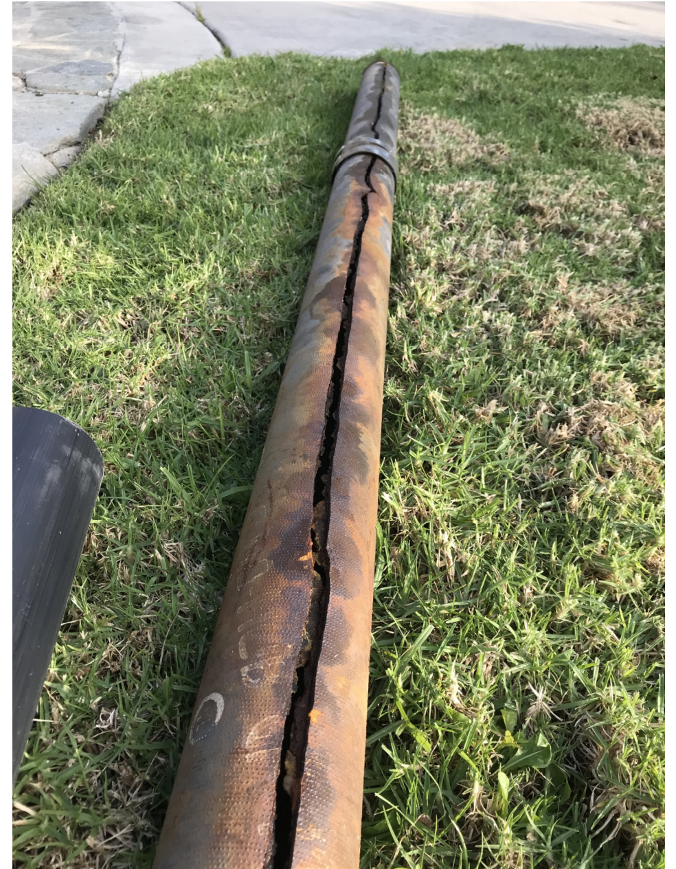
Typical Tru Spun Pipe Failure
