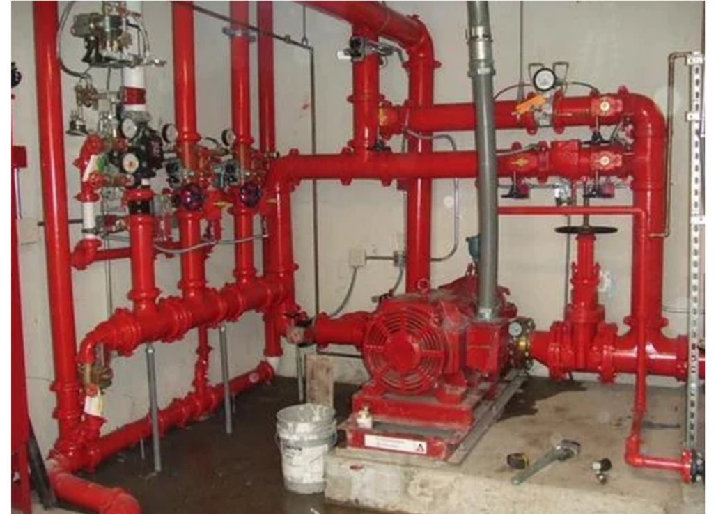
Electric Motor Driven Fire Pump
